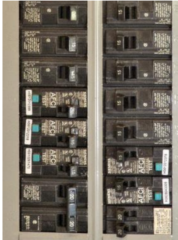
Figure 6. Breaker Box Equipped with GFI Breakers.
